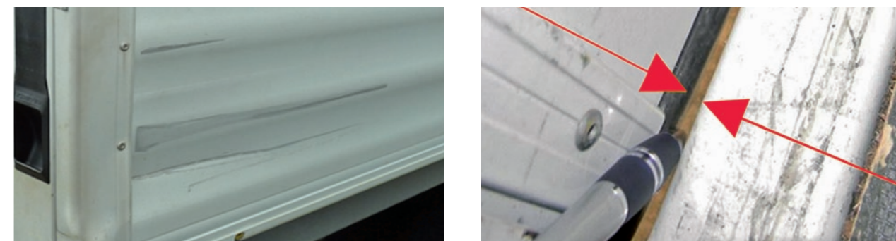
Deformations in the body closures not beyond economic repair, closure not possible or not sand-proof
