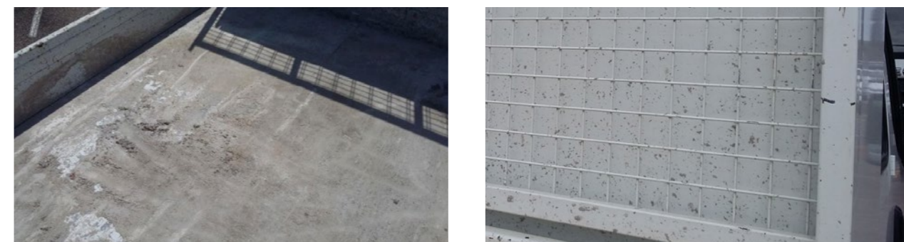
Trace of concrete or chemical product covering \geq 1/4 of the surface of the bed
