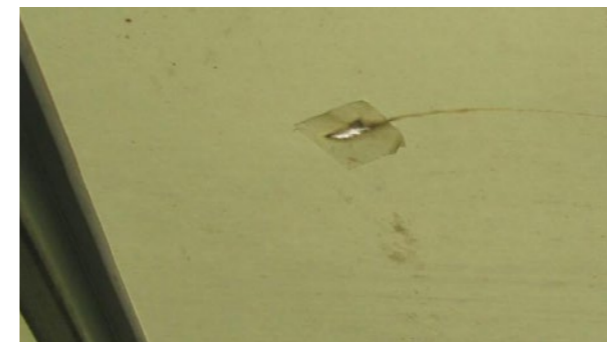
🔧 Roof space: Perforated or torn within economic repair
