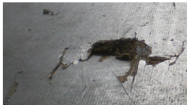
🔧 Flooring: Deformations or perforations within economic repair
