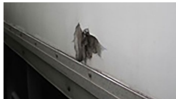
Wood side panels: Damaged wood support \geq 20\text{ cm}
