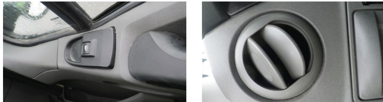
Slight decolouration due to sun exposure
