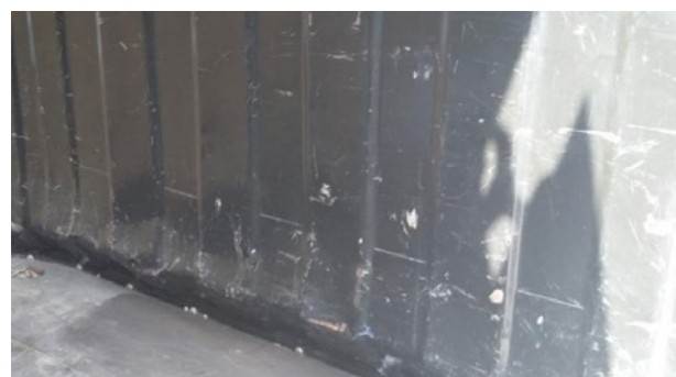
📅 Internal deformations: Slight deformation without perforations or cuts, repair time ≤ 3 h
